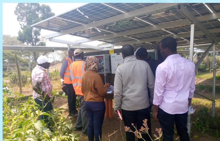
Site inspection and project progress meeting regarding the Solarization project by NAIVAWASCO team and Miale Solar team.
